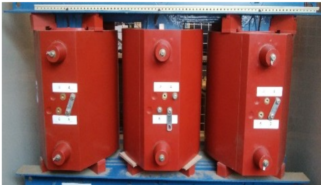
FIGURE 3. Research object transformer
