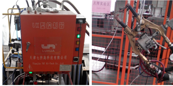
FIGURE 6. The control cabinet and welding tongs of the welding machine
